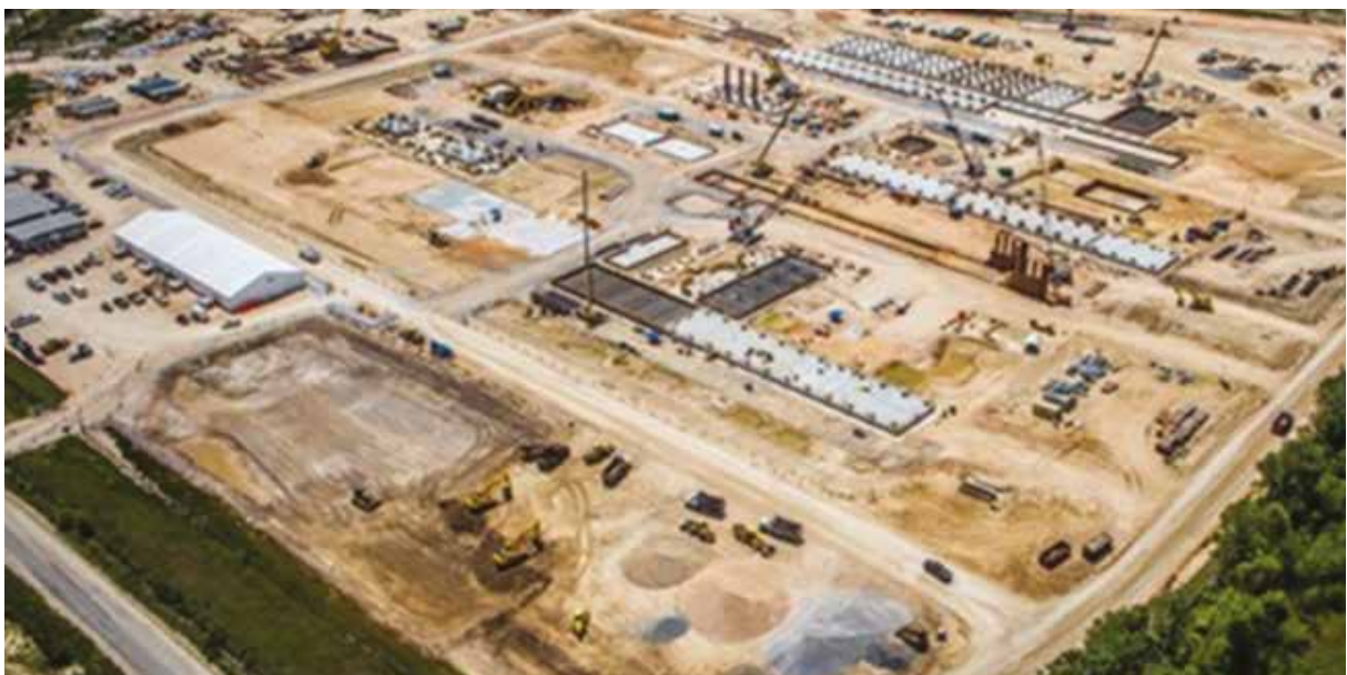
Lake Charles Chemical Project
